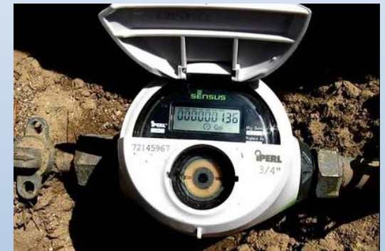
SFID water meter & shut-off valve
